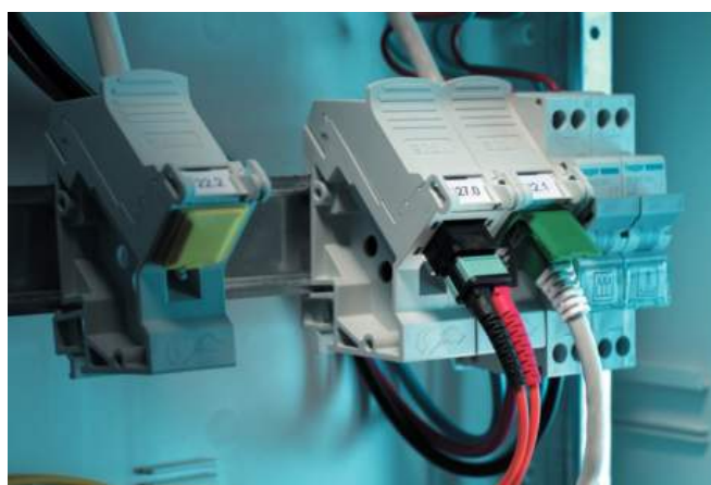
Figure 59: OTO integrated in the home electrical distribution panel
