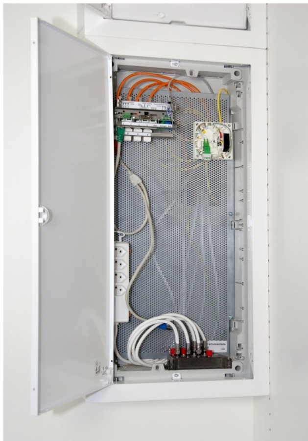
Figure 58: OTO integrated in a home distribution cabinet
