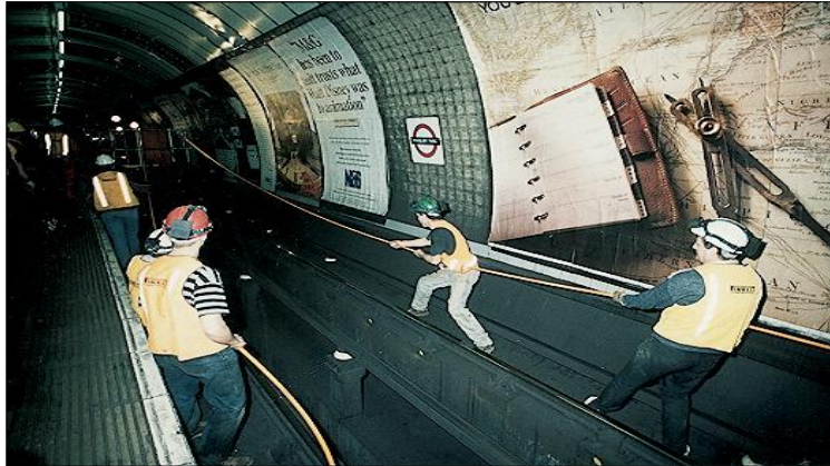
Figure 87: Cable installation in a train tunnel
