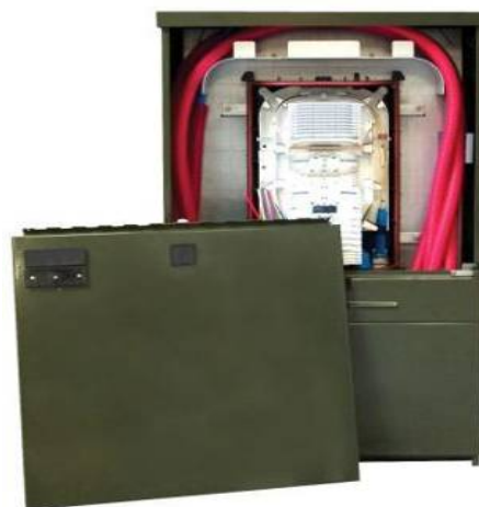
Figure 109: Typical street cabinet
