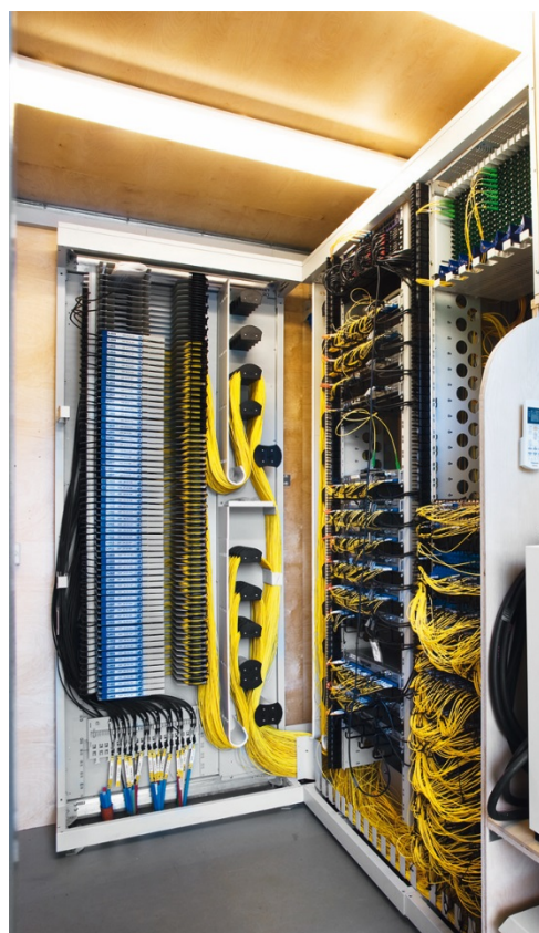
Figure 30: view into a POP equipped with an ODR, Ethernet switches, climate control and UPS.
