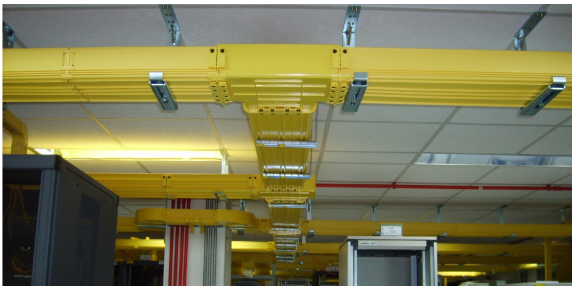
Figure 106: Examples of overhead fibre containment
